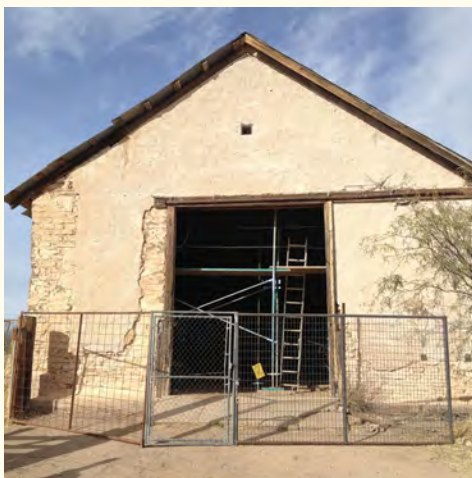
Adobe Haybarn security fencing and scaffolding herald the start of onsite stabilization work. (photo: A. Bunting)
