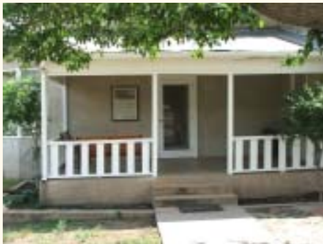
Volunteers at work repairing the front porch railing (photos: C. Auerbach, K. Patterson).
