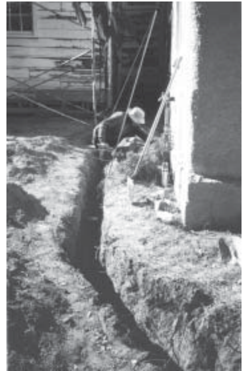
Electrician Xavier Valles prepares area where conduit will exit from south wall of Room 18.
