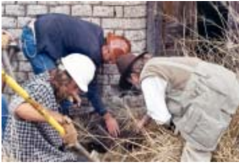
BLM Archaeologist Max Witkind (r) monitors excavation work for shorings on ranch hand's house west wall.
