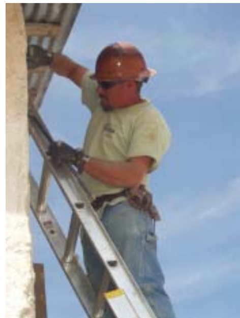
A Means Design crew member ties down the adobe haybarn roof to a straightened south wall. (photo: B. Lehmann)
