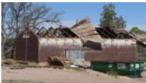
Recent wind damage to Mechanic's Shop (photo: BLM)
