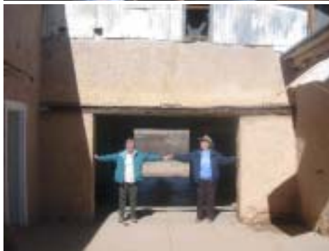
Zagan temporary shorings go away at last! Attic wall opening up high reveals the hidden steel now supporting the wooden lintel beams. (photos: C. Auerbach)
