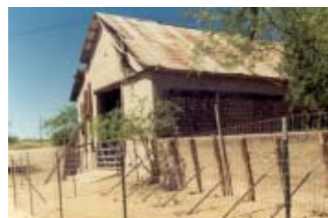
Adobe Haybarn awaits its turn for repair (Photos: T.Jover, L.Schupp)
