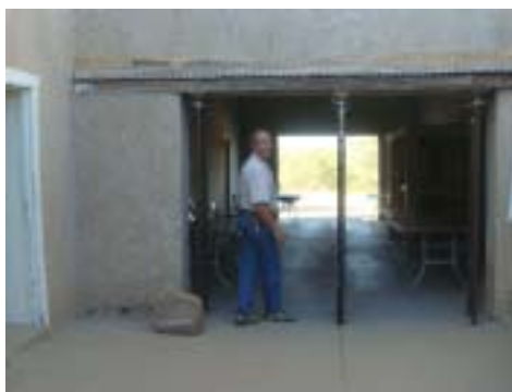
Repairs to the zaguan lintel are planned for 2008. Good riddance to those shoring posts! (photos: C. Auerbach, S. Hughes)
