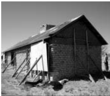
Adobe Haybarn beams and Hired Man's House braces were some of the conditions critically assessed in a recent structural assessment report by Statistical Research Inc. (SRI). (photos: SRI)
