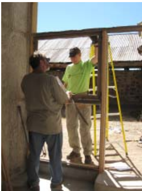
C. Schrager and R. Dirks repair partition at entrance to zaguan hallway (Stone Corral in rear). (photo: A. Bunting)
