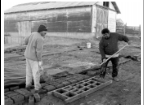
J. Egurrola and F. Montano of Means Design fill an adobe form. (Photo: SRI)
