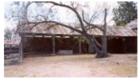
Stone Corral (north view): roof, support posts, walls and foundations are our next major project. (Photo: L. Wilkening)
