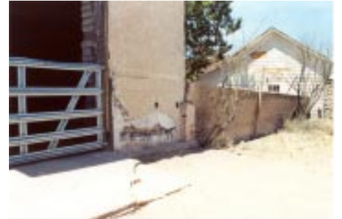
Adobe haybarn and adjacent concrete wall (southeast view): emergency shoring planned until preservation repairs to secure haybarn foundations and upright leaning wall (Photo: M. Witkind)
