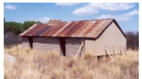
Ranch Hand's House (southwest view): will receive additional emergency shoring until preservation plan and repairs. (Photo: L. Wilkening)
