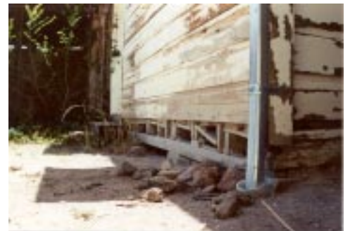
Children's Addition (northeast corner view): deteriorated wooden floor foundations need repair and stabilization (Photo: M. Witkind)
