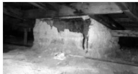
Perilous chimney foundations were identified in SRI's research for Action Plan . Repairs couldn't wait. (Photos: SRI)
