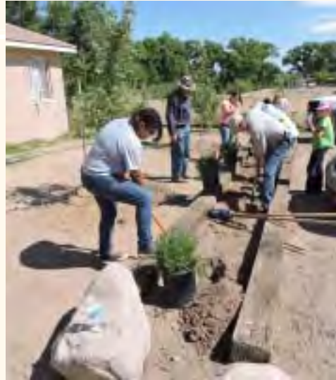
Volunteers, including Pascua Yaqui youth, plant shrubs in front of the VCS. (Photos: C. Auerbach)
