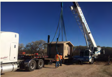
Restroom building lifted to allow site elevation to mitigate erosion (photo: J. Tayon)
